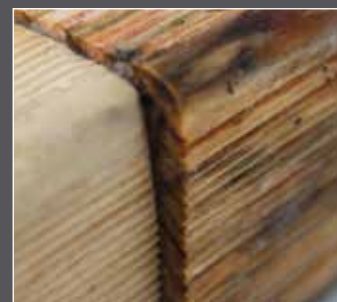
Swollen timber (right) unable to dry.
